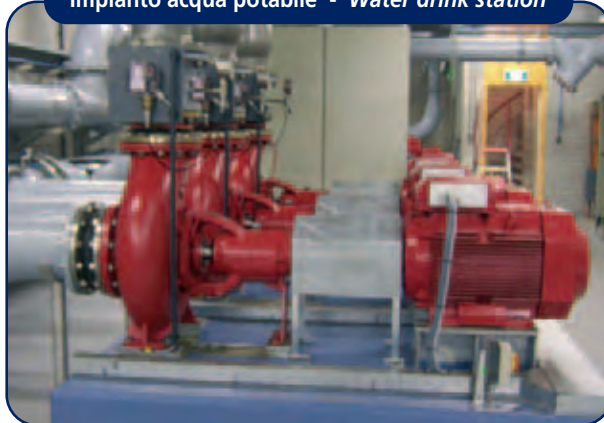
Impianto acqua potabile - Water drink station
